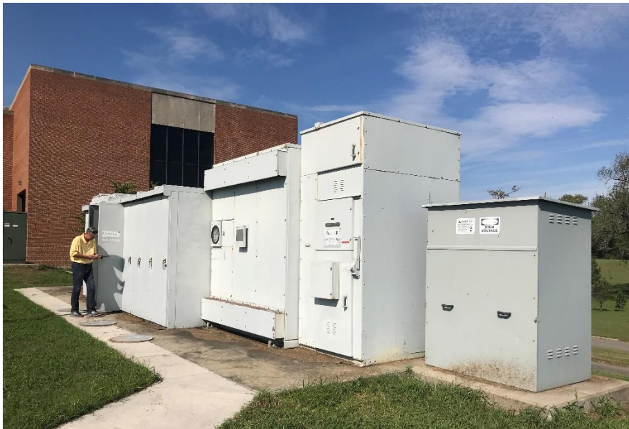
Unit Substation with Transformers T11 and T12 (FL EL. 34'-0")
