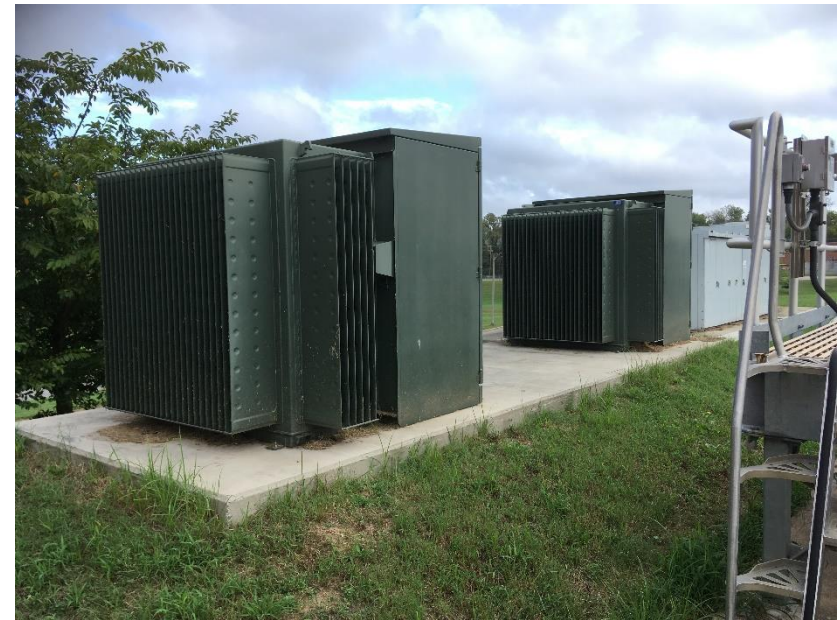
Transformers T2 and T21 (FL EL. 36'-0")
