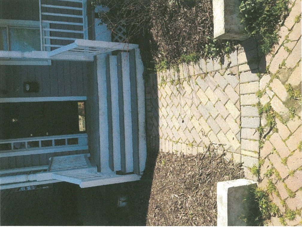
Existing walk way. Will be graded to zero degrees to allow the swing of the metal gate. This will create a 22" drop which will be addressed by adding two new steps.
