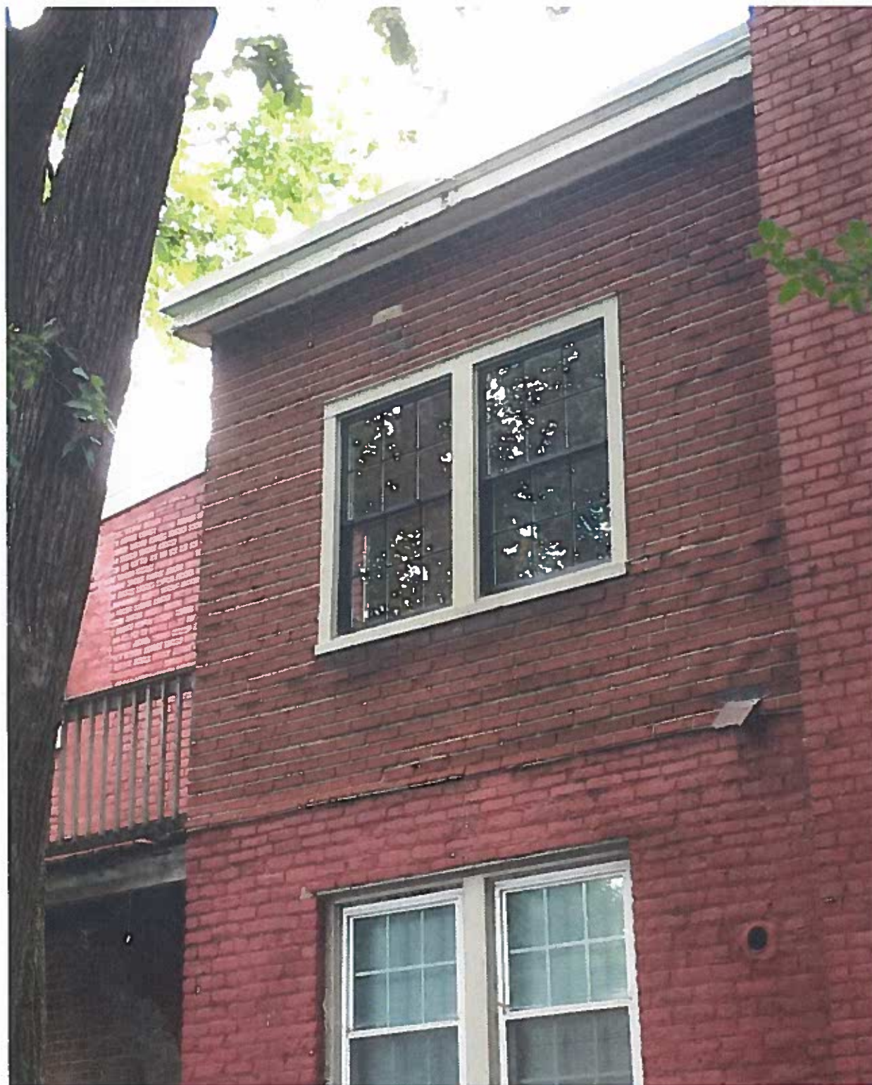
View of asphalt siding above brick wall, to be removed and replaced with wood clapboard.
