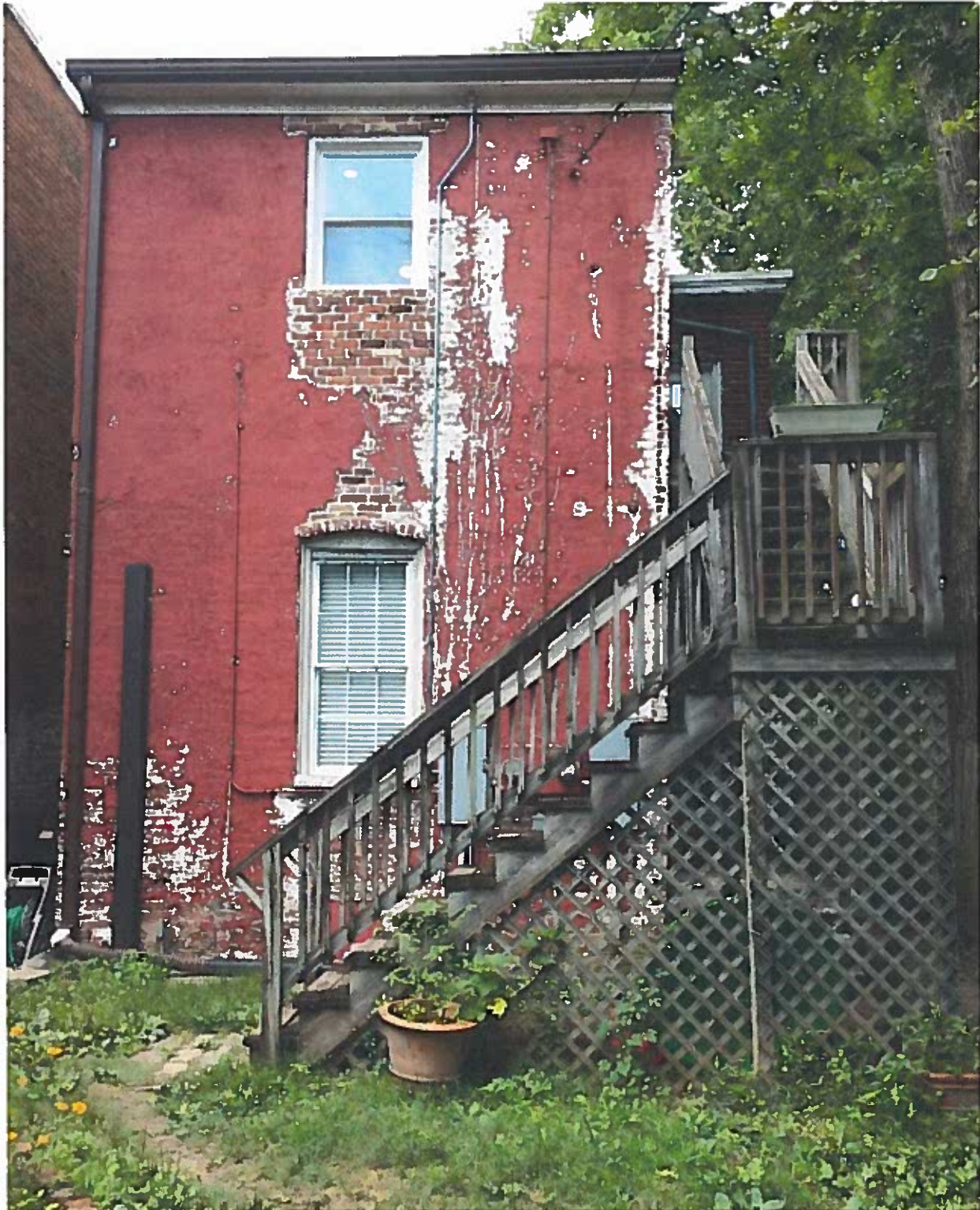
View of rear elevation facing alley between Broad Street and Grace Street.
