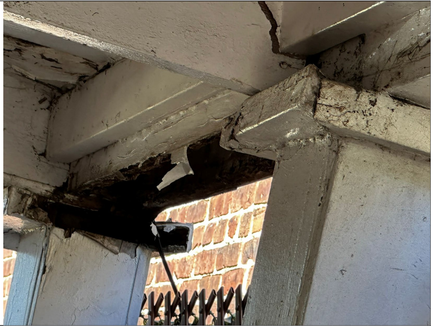
Close up view of the wood rot.
