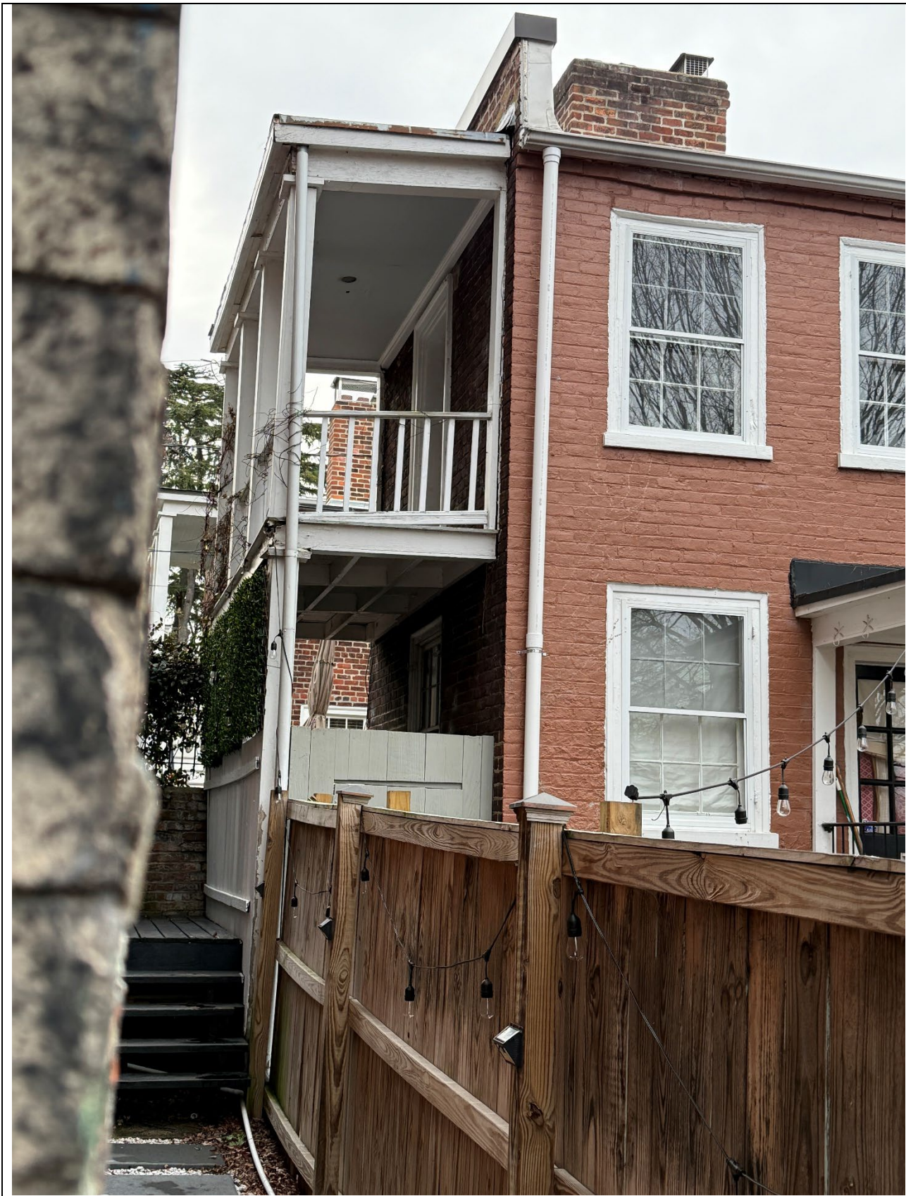
The view from 26th Street shows the sagging deterioration of the porch.
