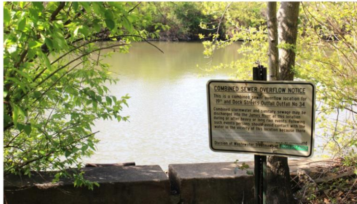
A combined sewer overflow outfall on the James River near downtown Richmond. (Sarah Vogelsong / Virginia Mercury)
