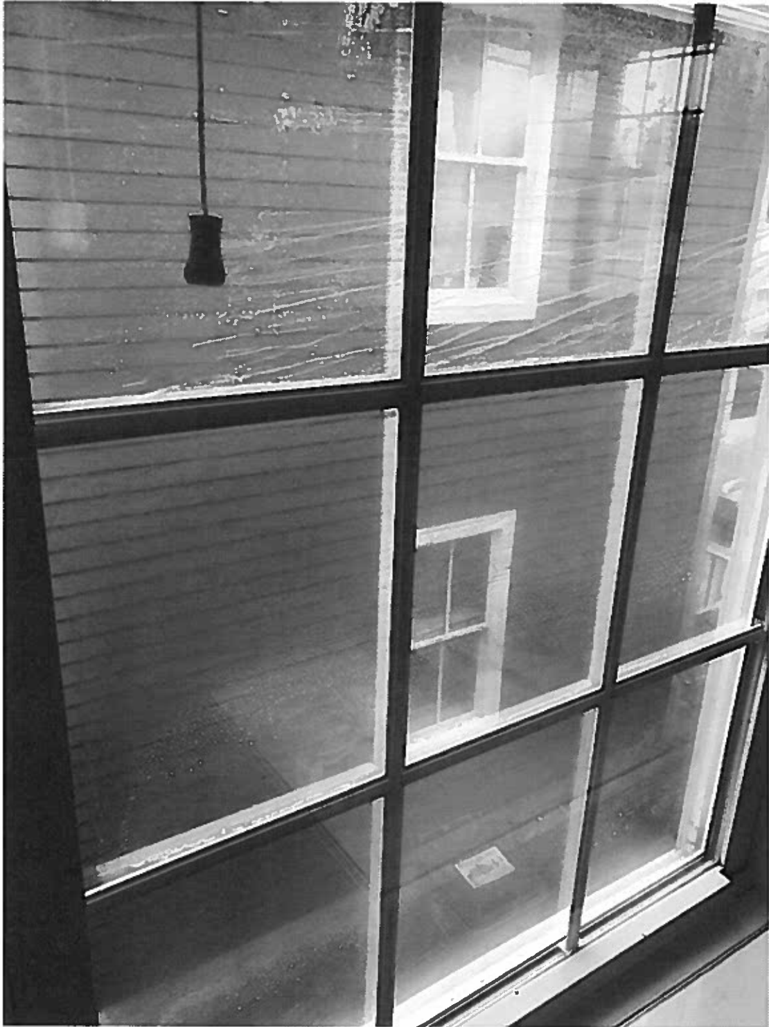
Window 4 Close up view of fog buildup on window pane due to seal failure
