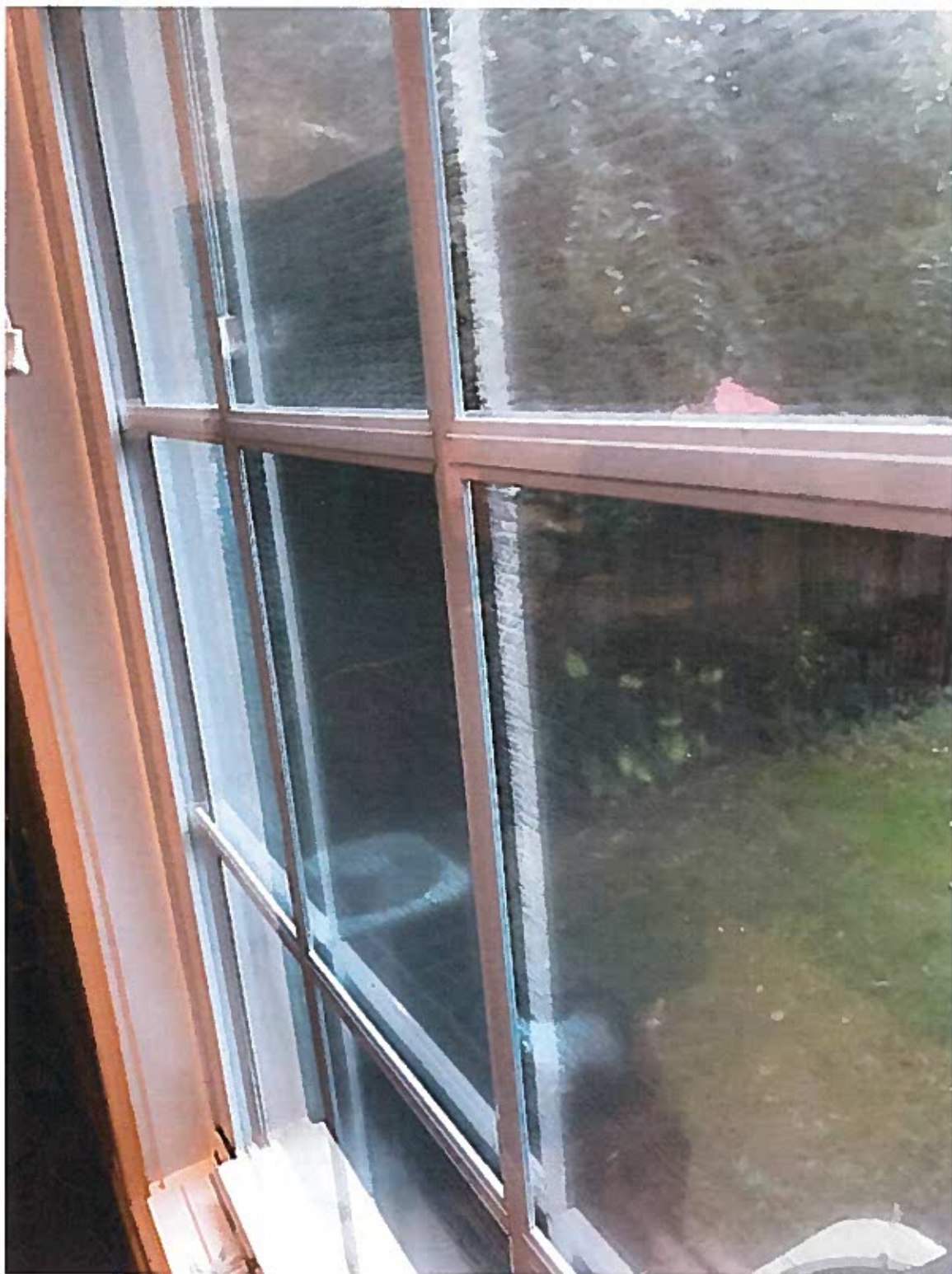
Window 5 Close up view of fog buildup on window pane due to seal failure
