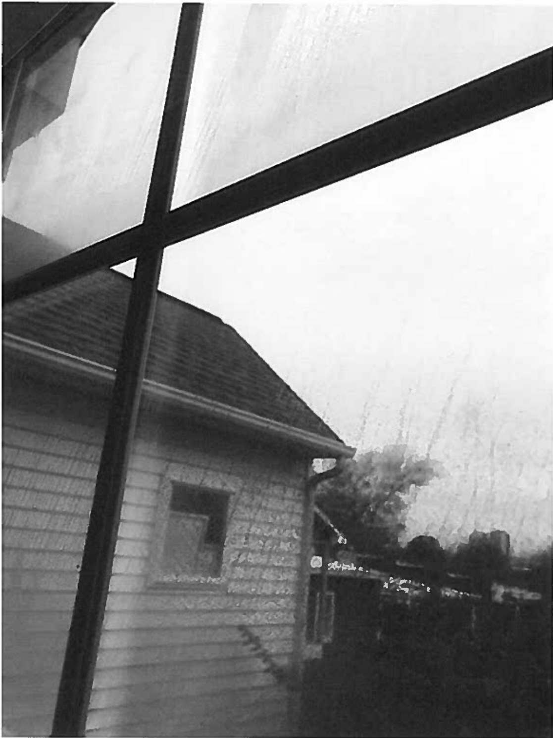
Window 7 Close up view of fog buildup on window pane due to seal failure
