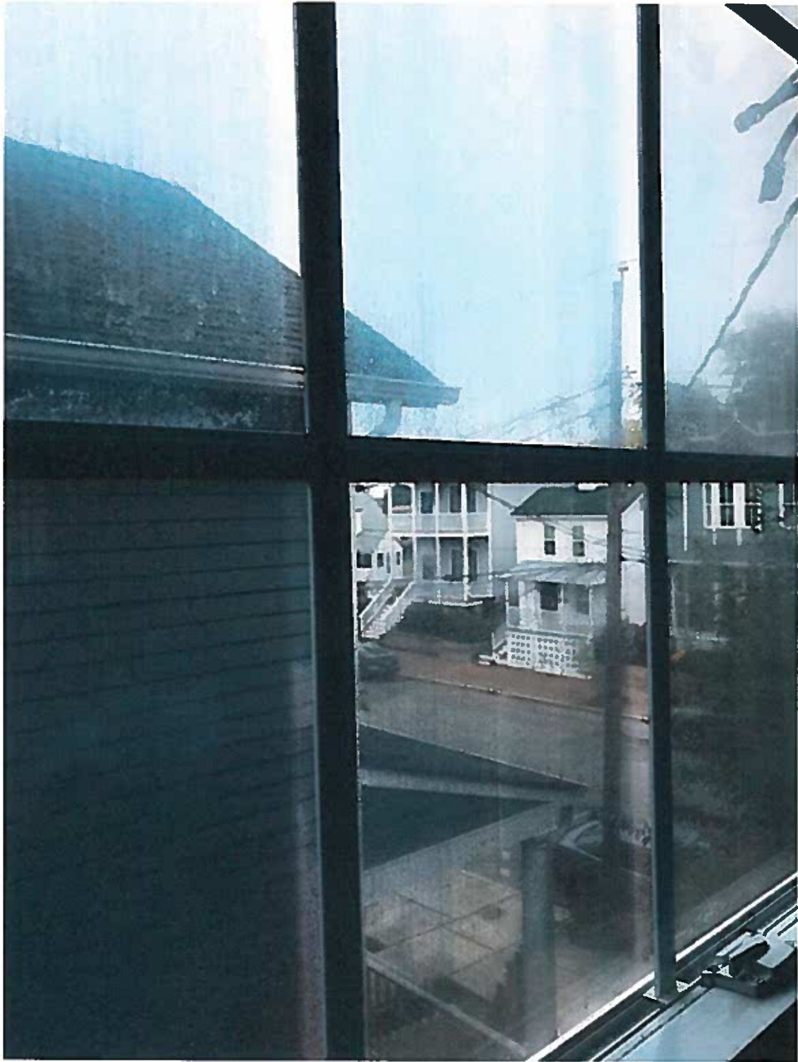
Window 3 Close up view of fog buildup on window pane due to seal failure
