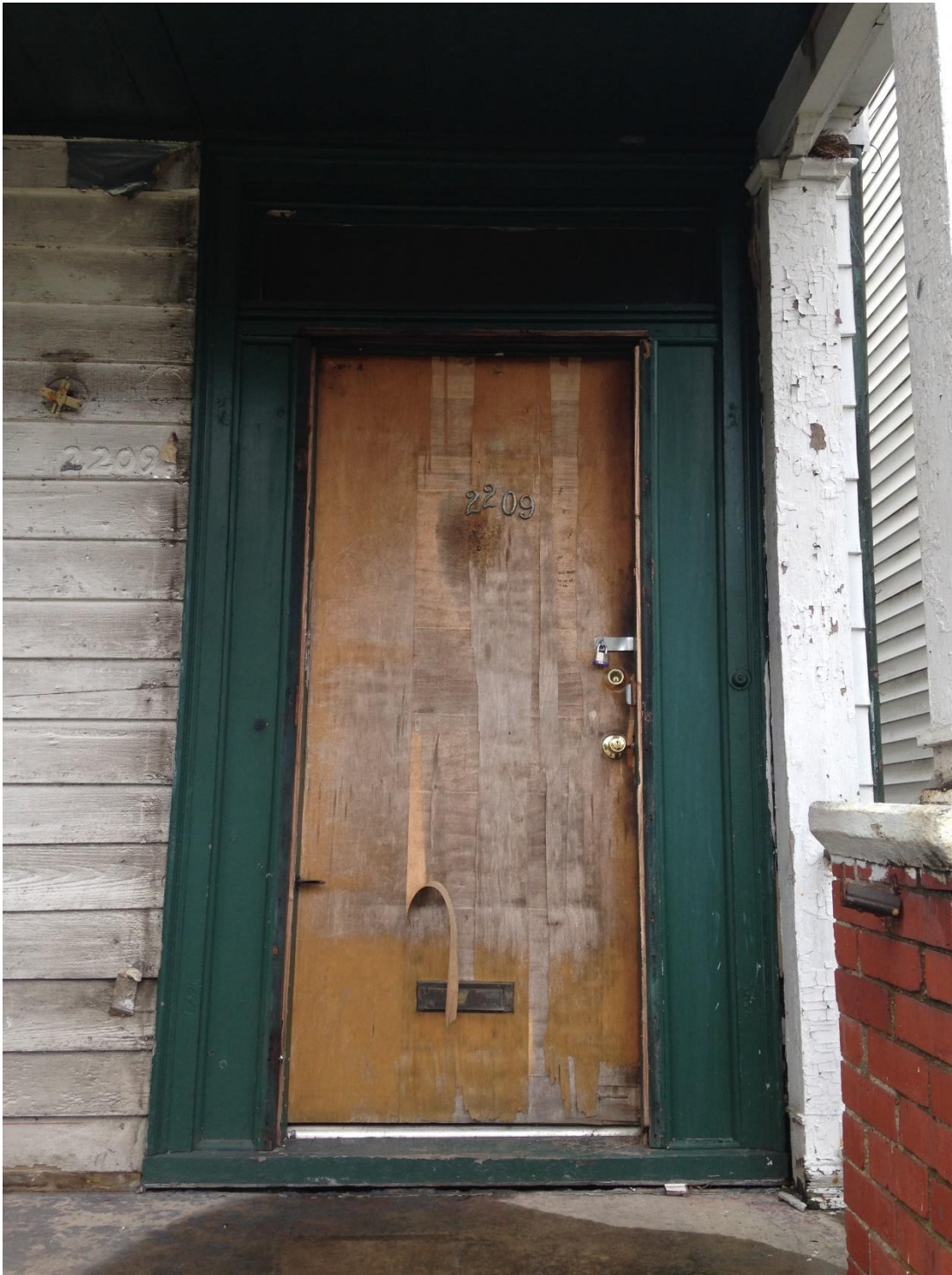
2209 Venable Street front door existing conditions.
