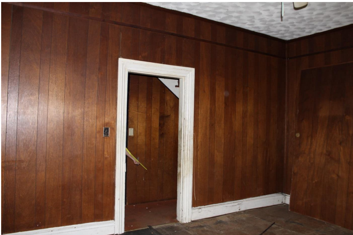
18. First floor rear room looking to the side hall, view to the northwest
