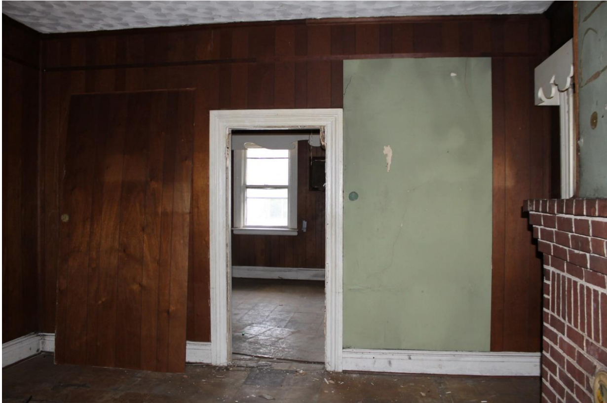
17. First floor rear room looking to the front, View to the north
