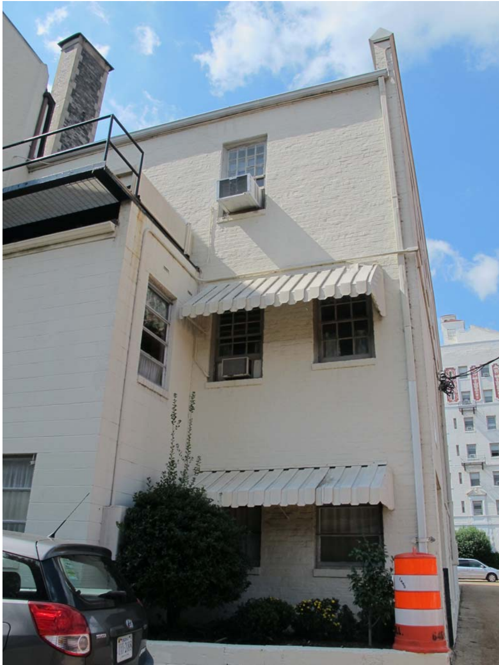
H. Rear wing with 2 ACUs to be replaced
