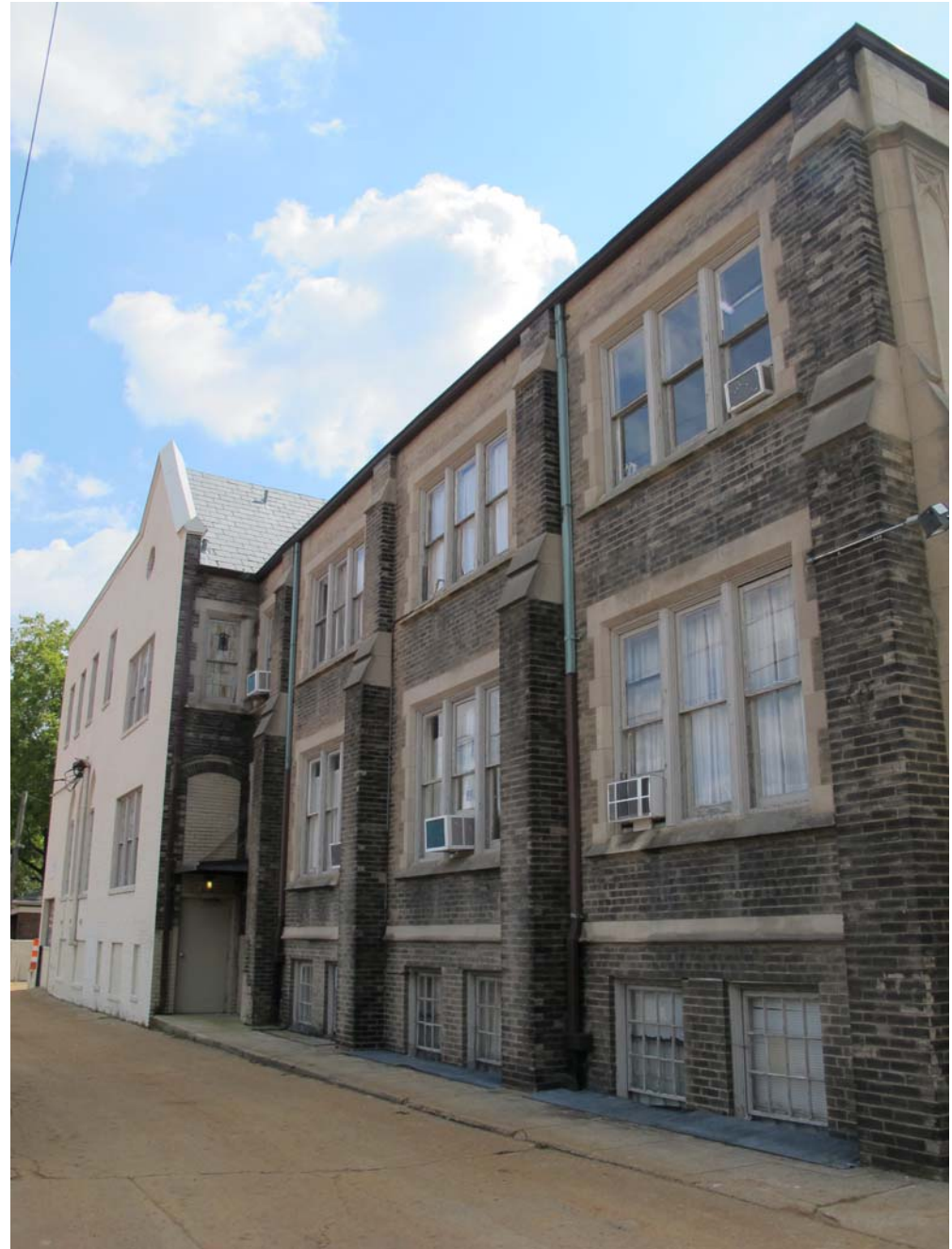
I. Alley view showing ACUs to be replaced (2 are missing)
