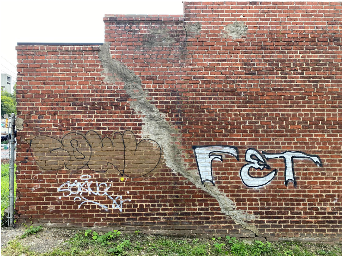
9a. Detail, masonry damage and inexpert repairs
