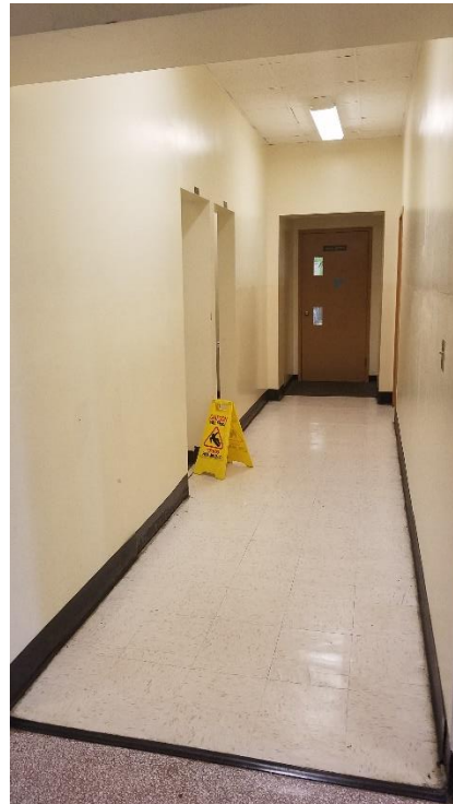
Figure 11. Non-ADA compliant bathroom corridors and spaces, ca. 1922 section. .
