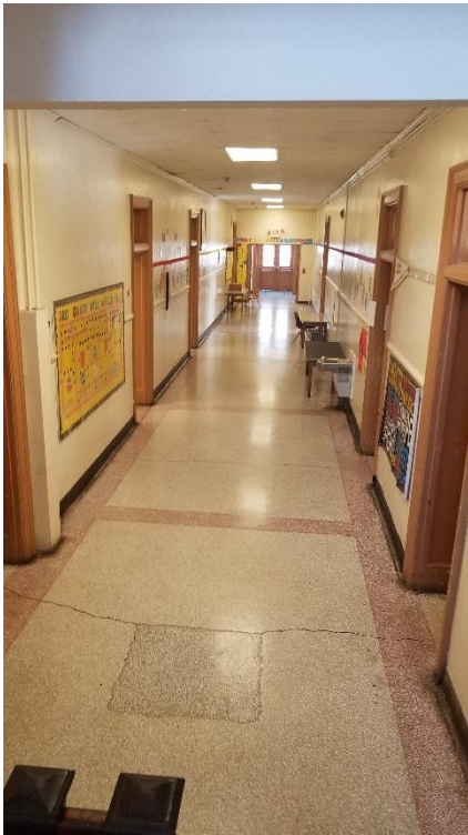
Figure 10. Cracking terrazzo floors, 1922 section.
