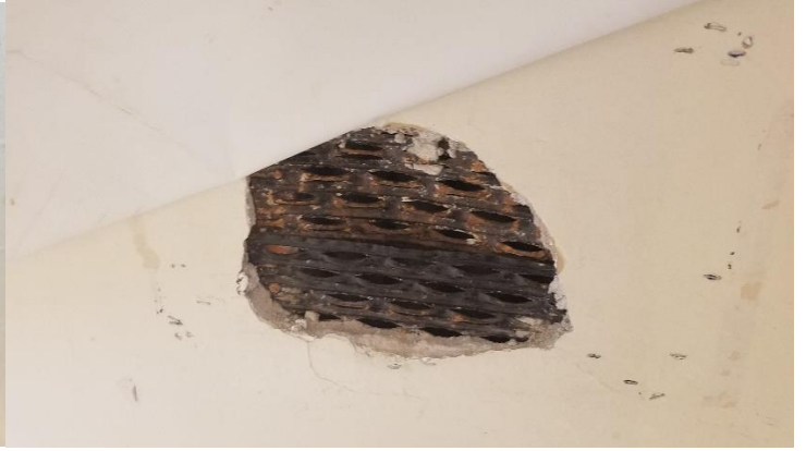
Figure 13. Damage to walls, ca. 1922 section.
