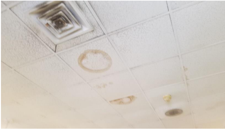
Figure 12. Extensive water damage observed on the ceilings.
