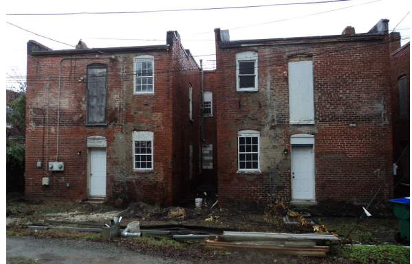
Figure 2. Rear of 3305-3307 East Marshall Street, CAR Files, 2015. Original porches had been removed, however ghosting of original porches and the neighboring porches at 3309-3311 East Marshall Street were used as a reference.
