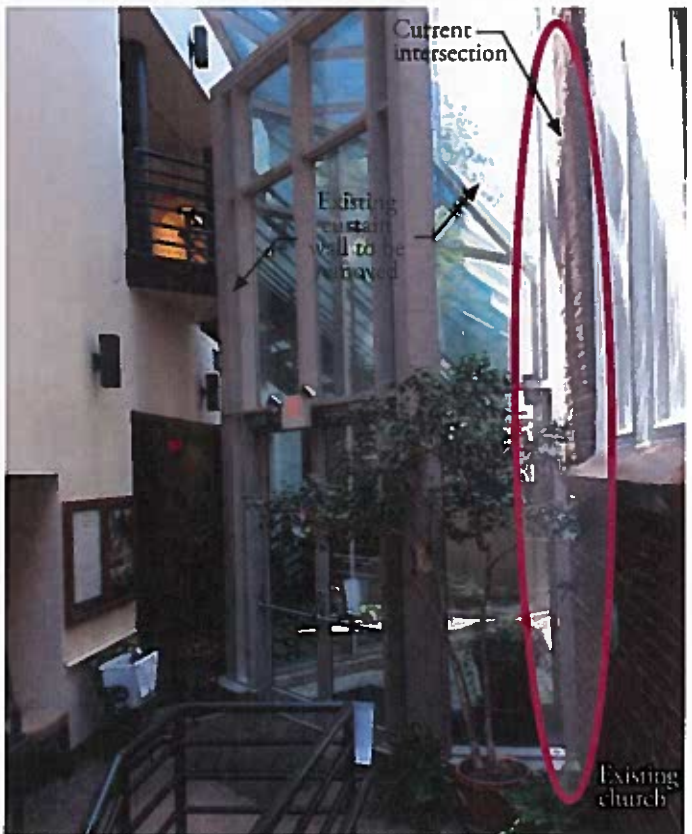
VIEW FROM INTERIOR LOOKING WEST AT EXISTING CURTAIN WALL CONFIGURATION AND INTERSECTION WITH EXISTING CHURCH
