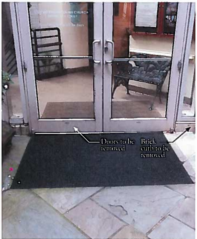
VIEW FROM COURTYARD OF EXISTING DOOR AND PAVERS TO BE REMOVED; BRICK CURB PROFILE TO BE REPLICATED AT NEW CURTAIN WALL SILL
