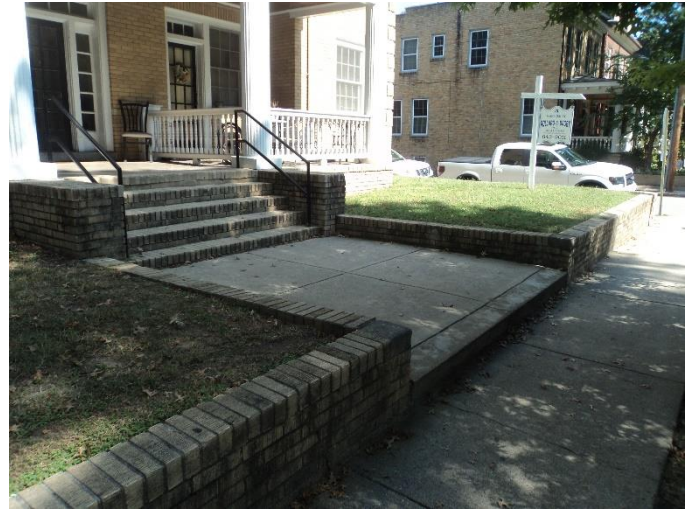
Figure 2. Example of a concrete walkway at an apartment building at 3000 Monument Avenue
