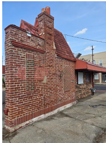
Figure 2. 1000 N 25 th Street –Previously infilled window openings on original portion of the building.
