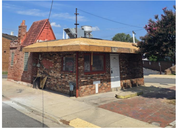
Figure 2. 1000 N 25 th Street – Repair to canopy underway and new glass block windows installed.
