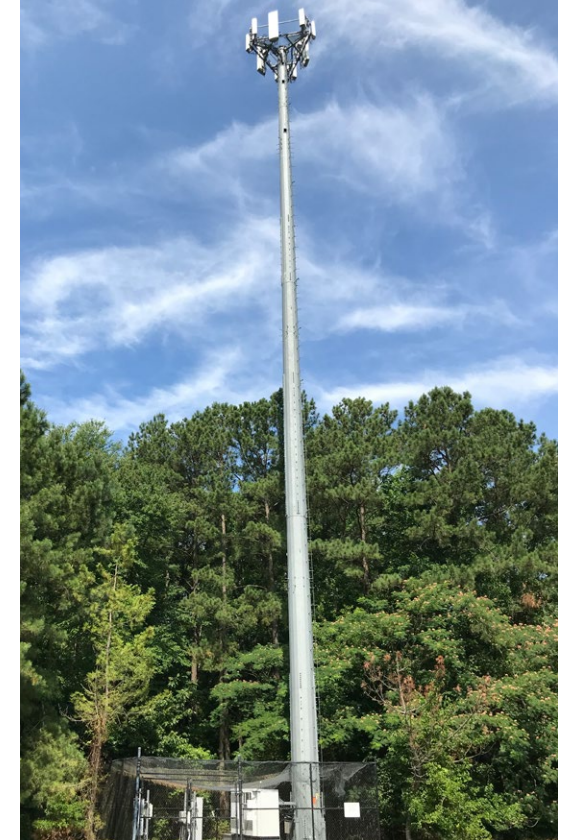
EXISTING CELL TOWER
