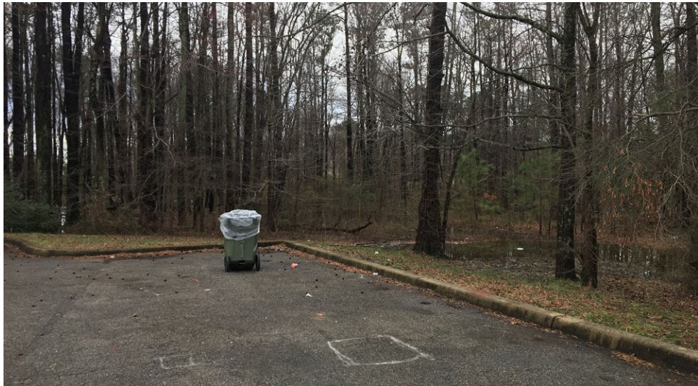
FRONT PARKING LOT DRAINAGE INTO LOW LYING AREA
