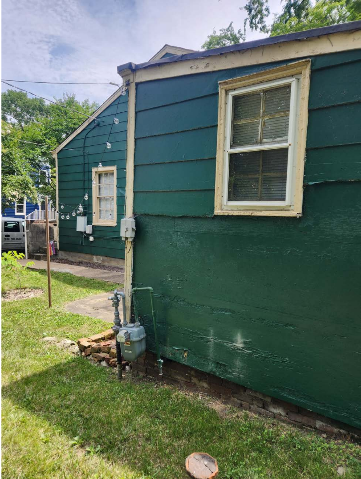
Image 7: View of right side of house (side D) from back right corner of property
