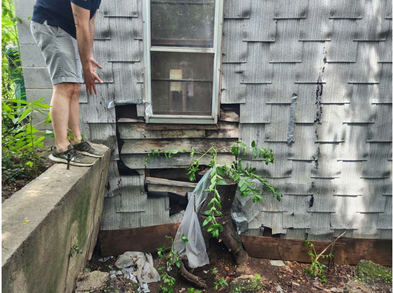
Image 9: Left side of house (side B) showing damage from an Ailanthus tree. This side of the house is a zero lot line and photo is taken from behind garage at 620 N 23rd St. This area is not visible from M Street, N 23rd St, nor the alley.
