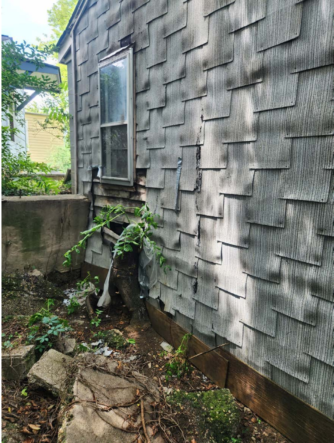
Image 11: Left side of house (side B) looking toward rear of house. The collapsing retaining wall on left sits between 616 and 620 N 23rd street and is not part of my property.
