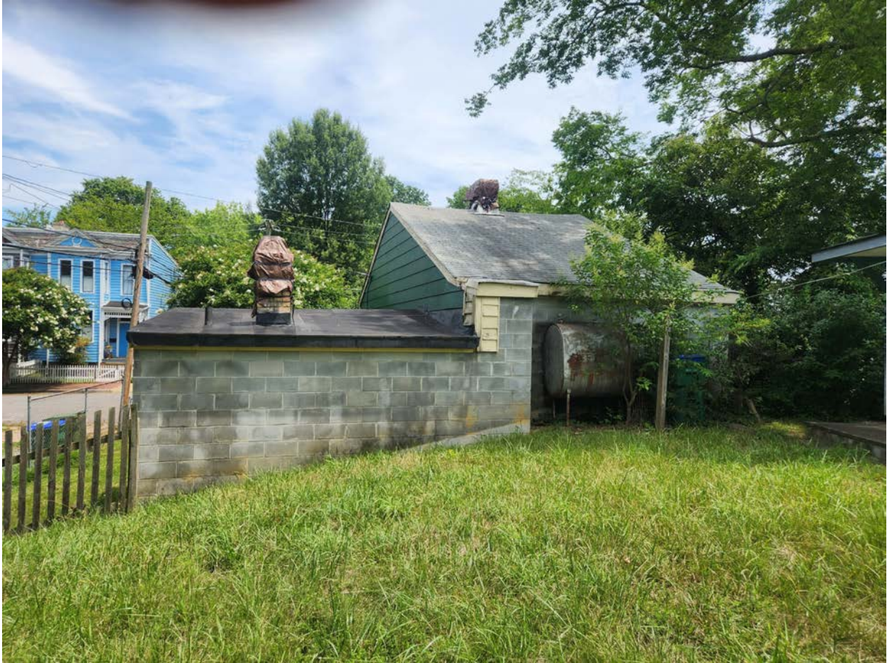
Image 8: Rear of house (side C) from rear yard of 616 N 23rd St. which is a zero lot line.
