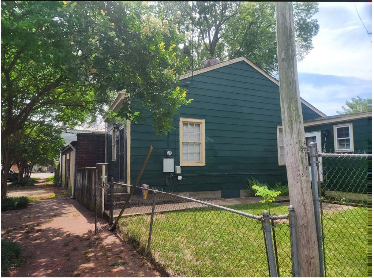
Image 4: Right side of house (side D) from property corner (M Street and Alley)
