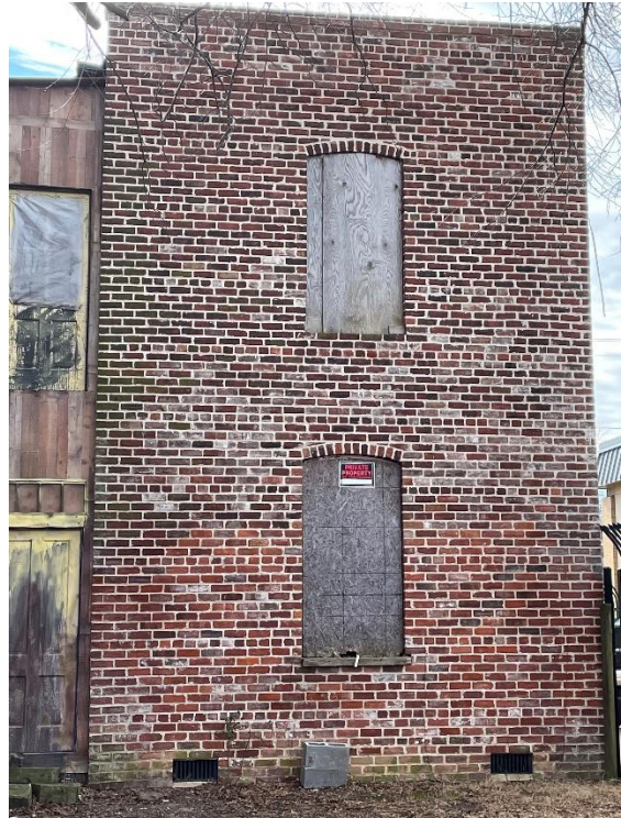
Figure 6. 316 W Leigh Street, rear windows.
