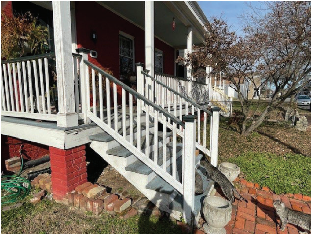
Photo #3: EXISTING CONDITION: Overall View #2 of front porch with existing Richmond Rail
