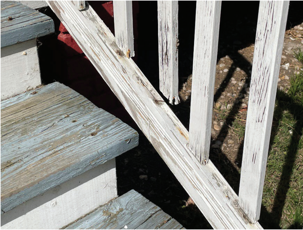
Photo #4: EXISTING CONDITION: Detail View #1 of Richmond Rail going up the front steps
