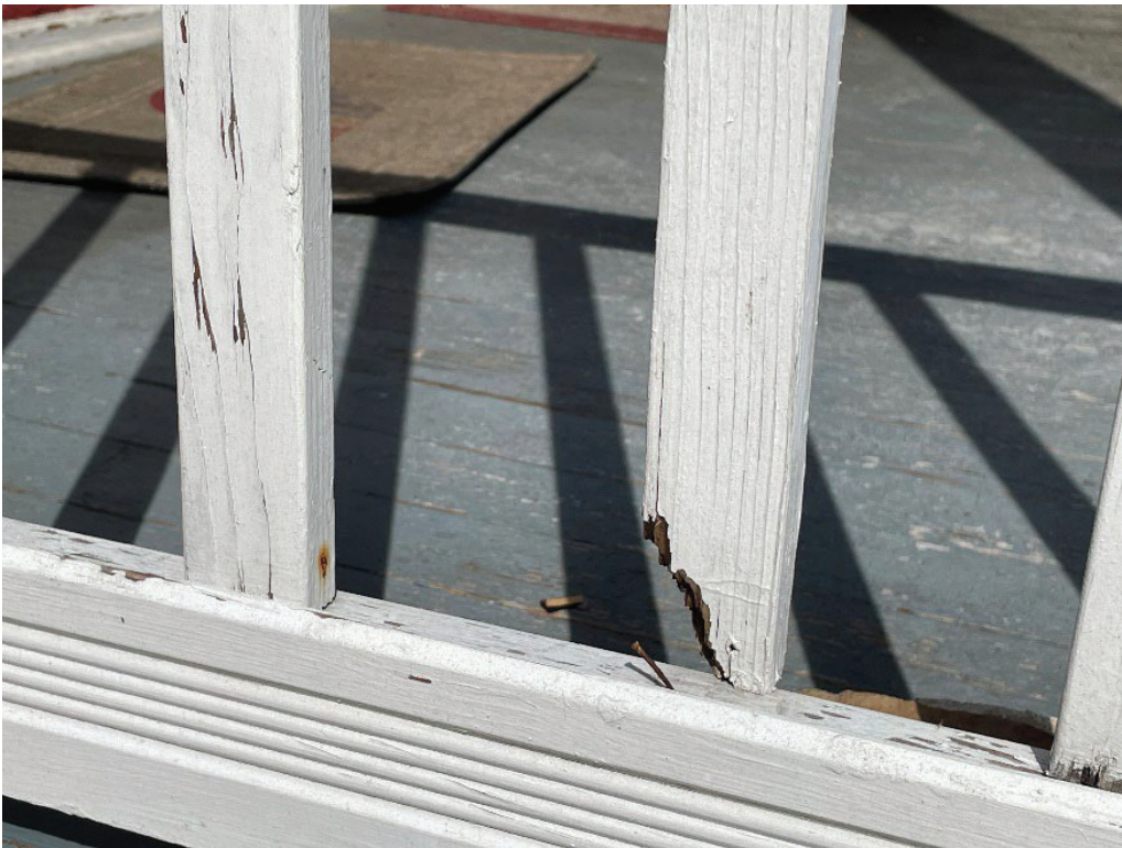
Photo #5: EXISTING CONDITION: Detail View #2 of Richmond Rail, south end of porch
