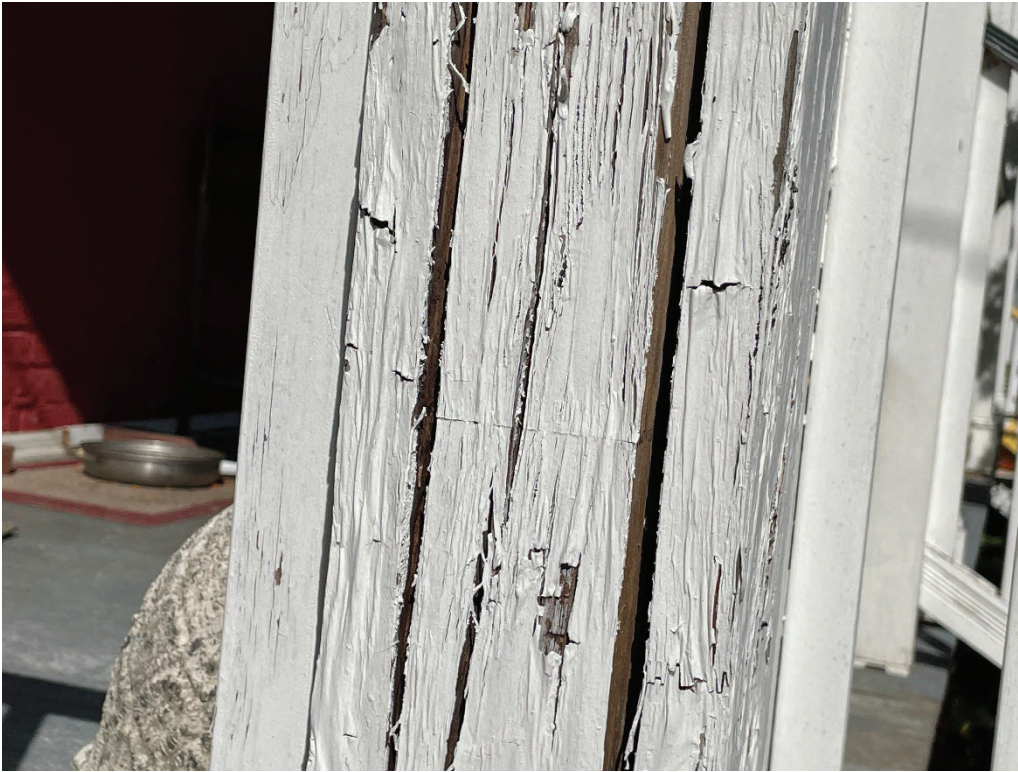
Photo #8: EXISTING CONDITION: Detail View #5 of deteriorating box column board, split open
