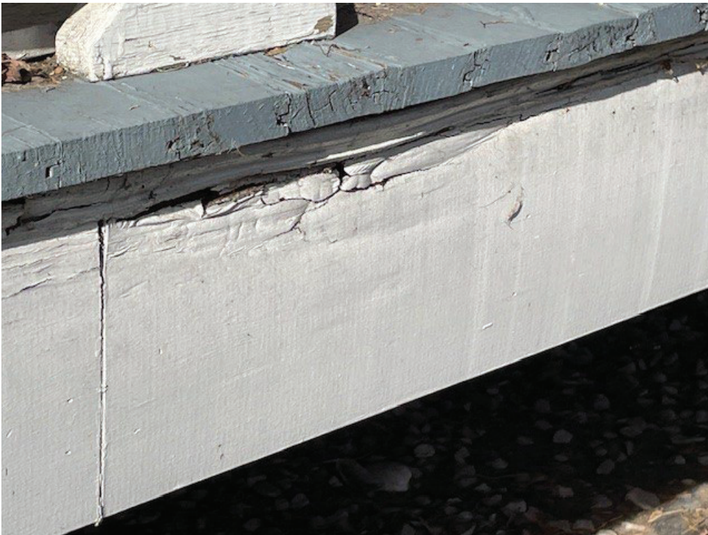
Photo #9: EXISTING CONDITION: Detail View #6 of deteriorating box column / base & porch fascia
