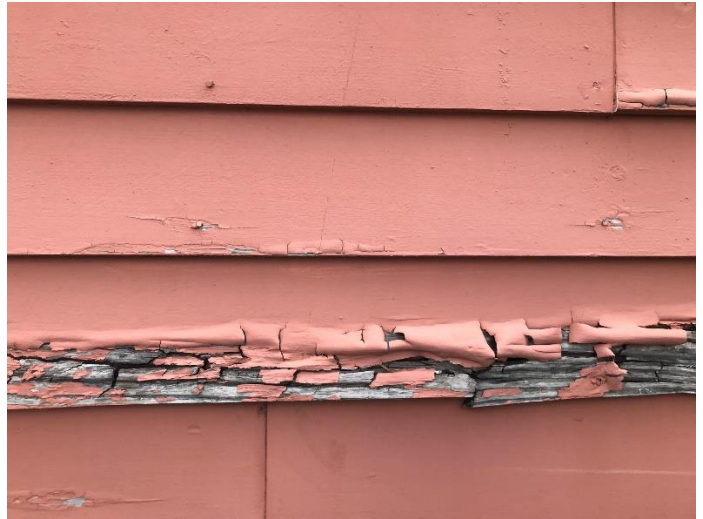
Figure 2. detail of damaged siding
