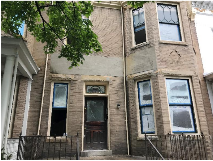
Figure 5. 2010 West Grace Street, porch roof ghosting.
