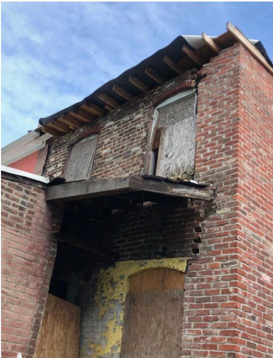
Figure 3. Structural damage at rear wall
