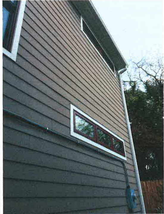
Example of three ganged horizontal windows (ours would not have the trim, and would be recessed); 601 N. 21 st Street
