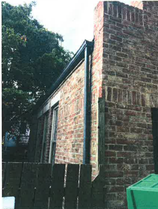
Example of gutter at roof edge of gable roof; 15 N. 29th Street
