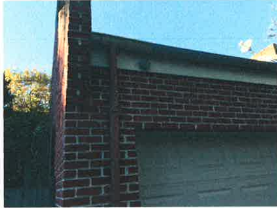
Example of gutter at roof edge and behind parapet; 11 1/2 N 29th Street
