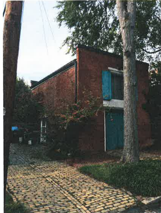
Example of metal parapet cap and roof edge gutter; 2717 East Grace Street
