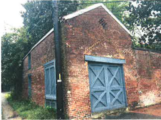
Carriage house with masonry gable end and gable roof; 2300 East Broad Street
