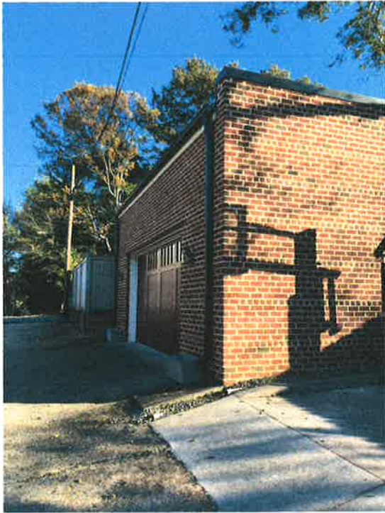
Examples of metal parapet cap, gutter without soffit, and downspout; 3516 East Broad Street
