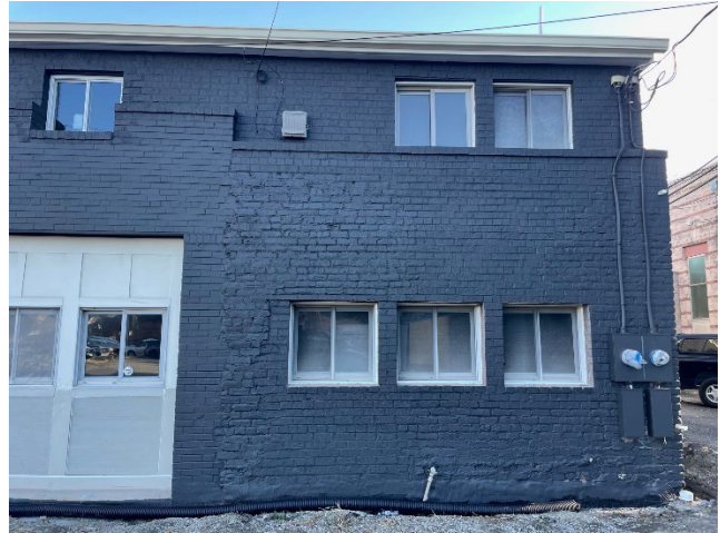
Figure 6. Existing Conditions, October 2023. New masonry openings added to the second floor and building painted a singular color. Three lower windows were completed as part of the 1994 rehabilitation.
