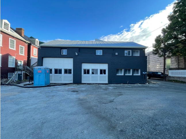
Figure 5. Existing Conditions, October 2023. New masonry openings added to the second floor and building painted a singular color.
