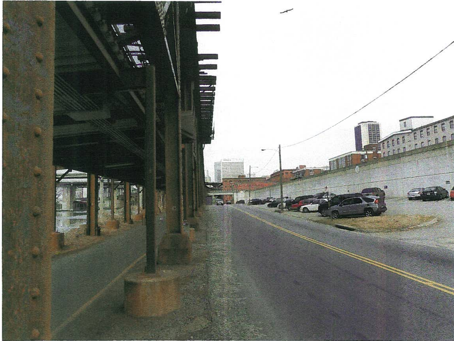
CAPITAL TRAIL (B) - EXISTING CONDITION
