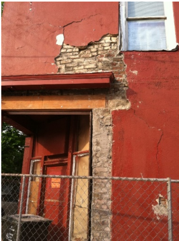
Figure 7. Deterioration around the door, April 2019.
