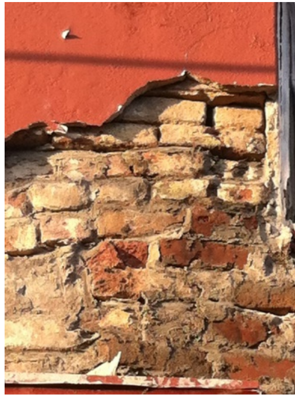
Figure 10. Detail, of additional deterioration, May 2019.
