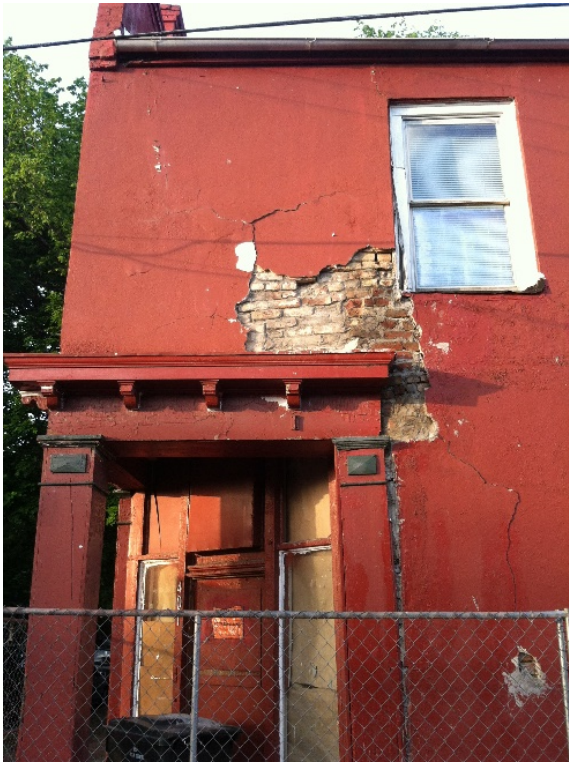
Figure 9. Additional deterioration, May 2019.
