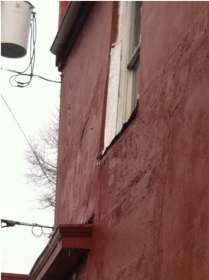
Figure 3. Evidence of cracking, January 2019.
