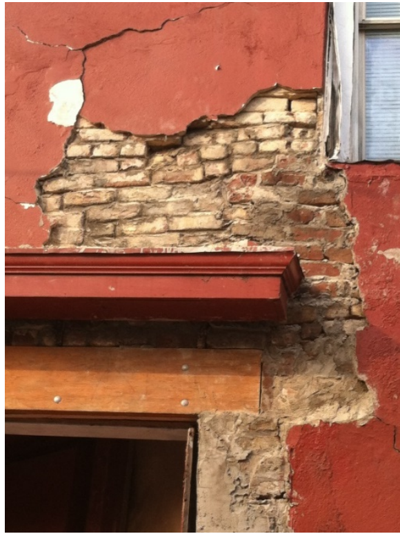
Figure 8. Detail of deterioration around the door, April 2019.
