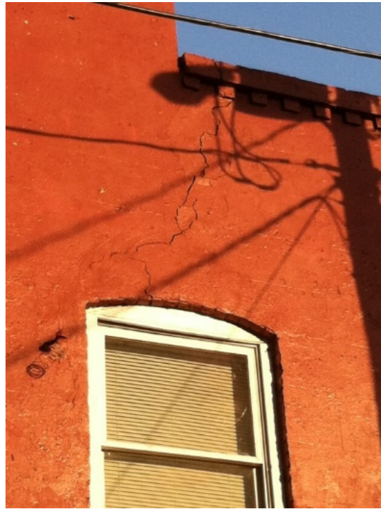
Figure 12. Detail of additional cracking on the west wall, May 2019.
