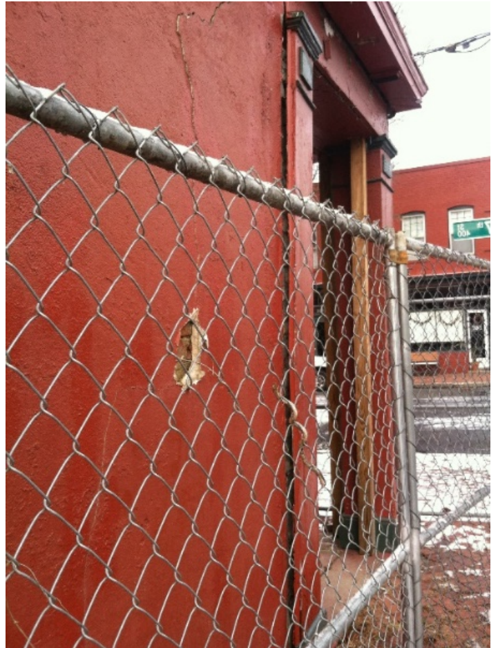
Figure 4. Hole and cracking, corner supports, January 2019.
