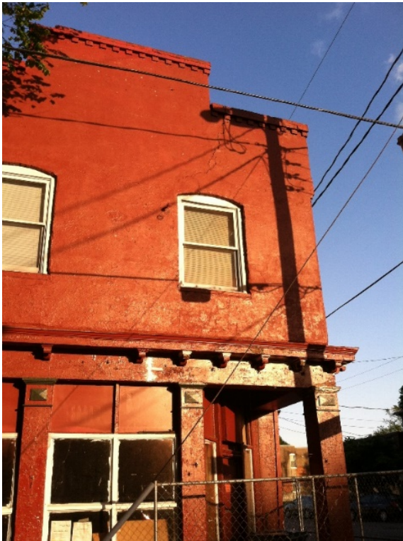
Figure 11. Additional cracking on the west wall, May 2019.
